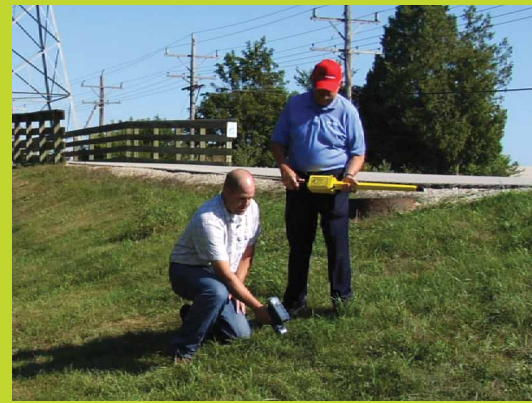
LaFond verifies an RFID marker location in a rural area while Bill Rushing, vice president of research and development for Berntsen, looks on.
